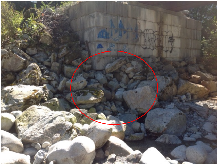
upstream left bank riprap scour - lock block scour
