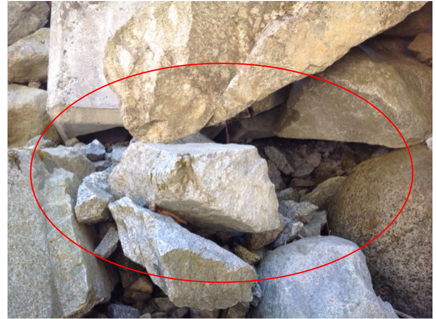
upstream left bank lock block (abutment scour)
