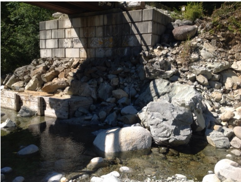
upstream right bank riprap scour
